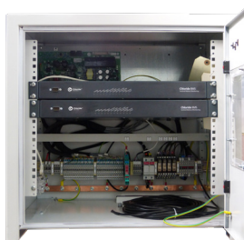
Chloride ® BMS Box with Controller modules installed
